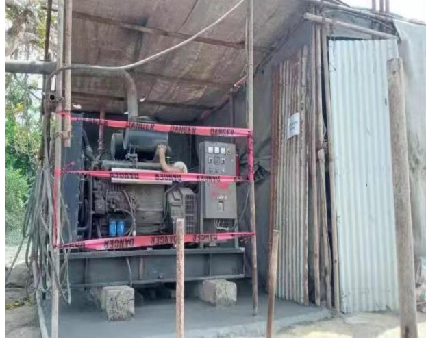
Image-7: Paved surface under Generator to check oil leakage in P-39/2C, Package-2
