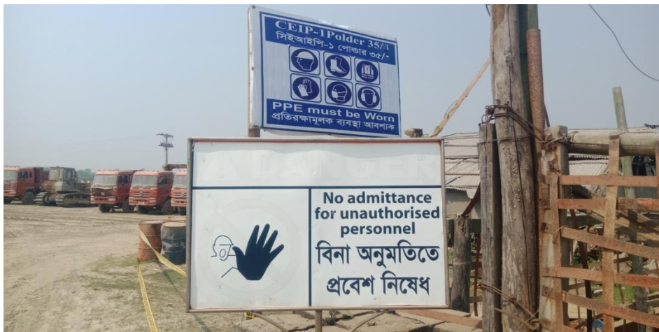
Image-5: Erected cautionary signboard in P-35/1, Package-1
