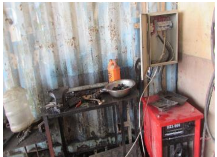
Electric box opened in the workshop
