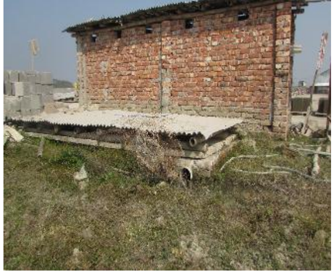
Septic tank of another latrine directly opened to drain inside plant yard
