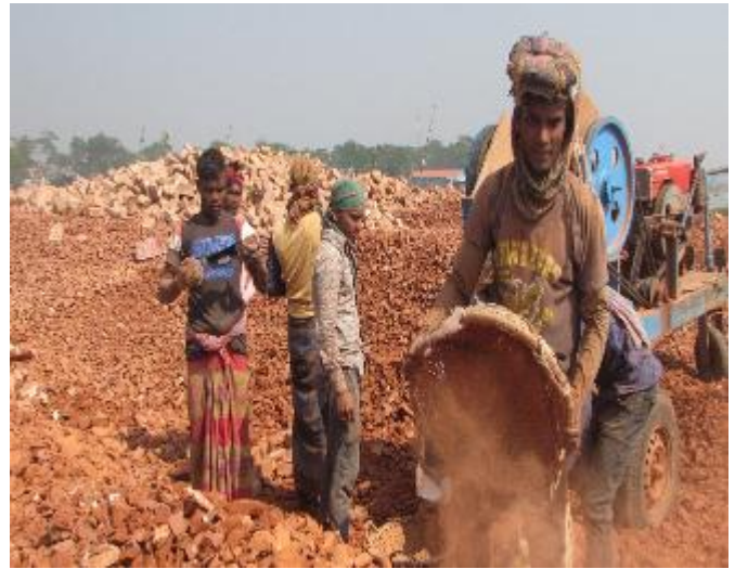
Workers without PPE
