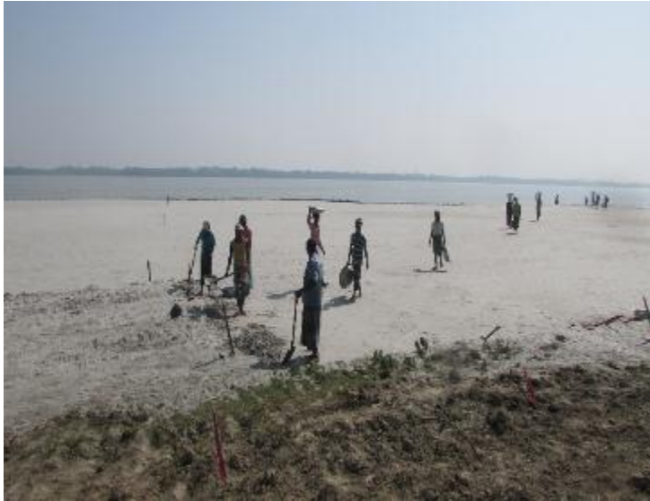
Workers working without PPE
