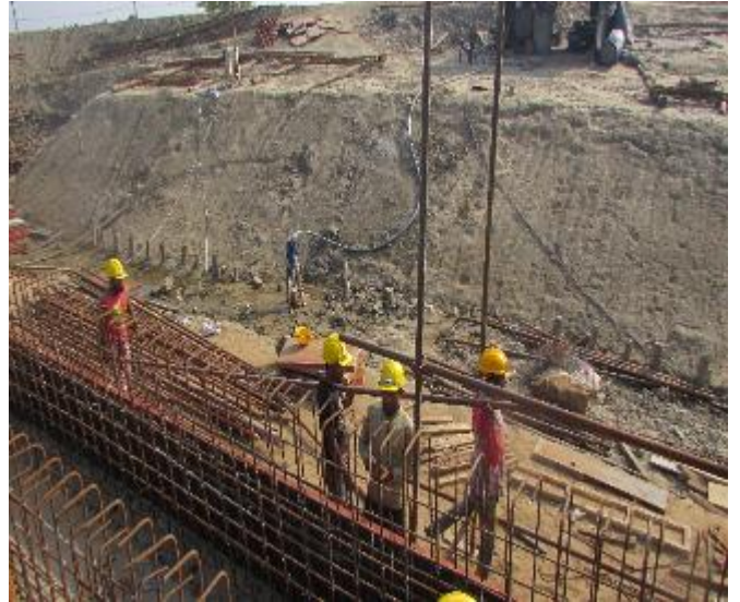
Workers dealing with heavy materials without hand gloves
