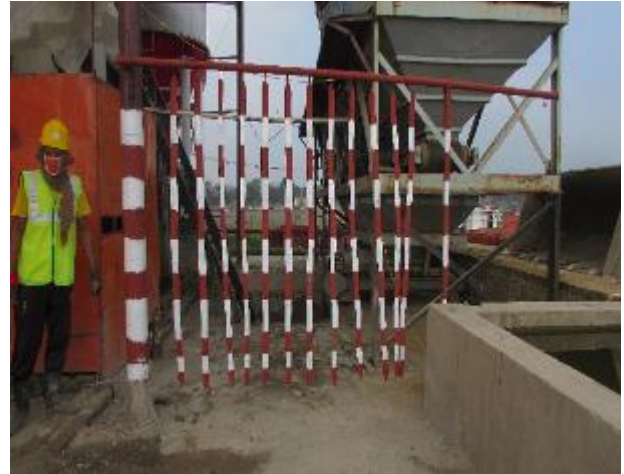
Cover over the conveyor belt of CC block manufacturing plant
