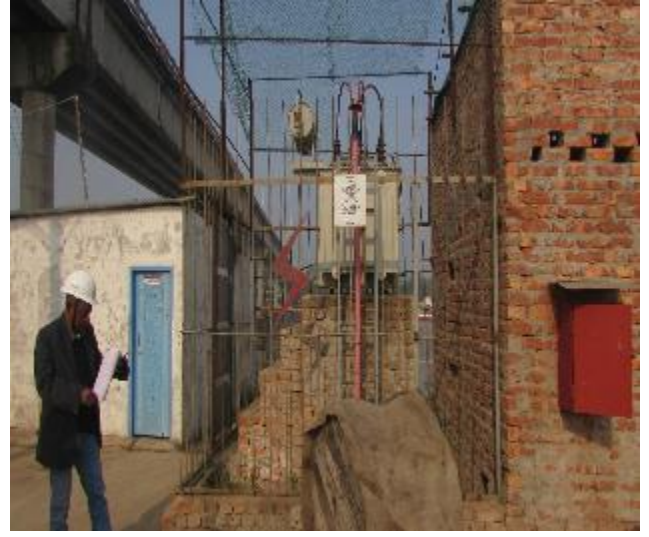
Well protected electric supply room
