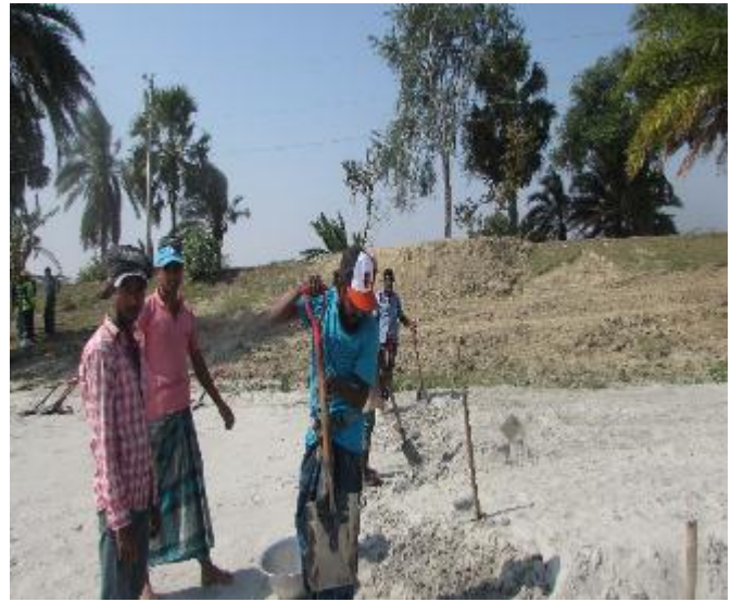
Workers working without PPE
