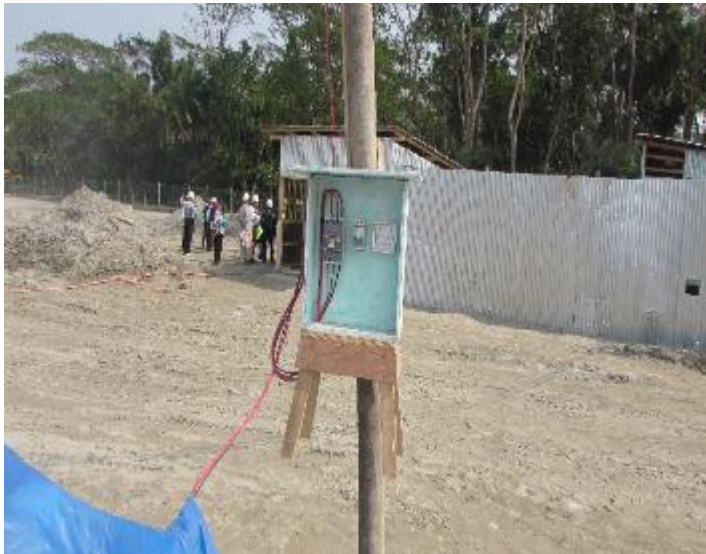
Opened electric board
