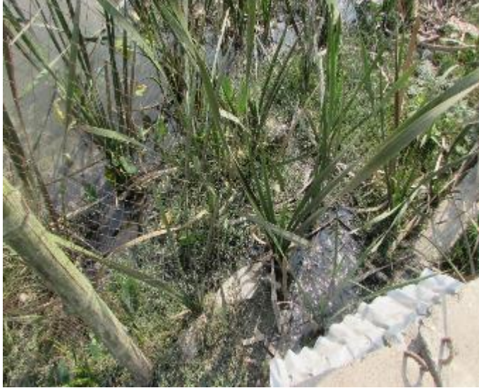
Septic tank opened to nearby ditch passing discharge
