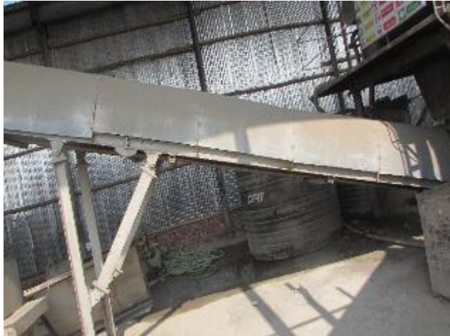
Moveable fencing has been provided around the pit Of left over materials of CC plant
