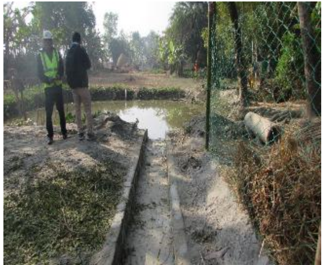
Drainage outlet from the work site directly opened to a pond used by community HHs
