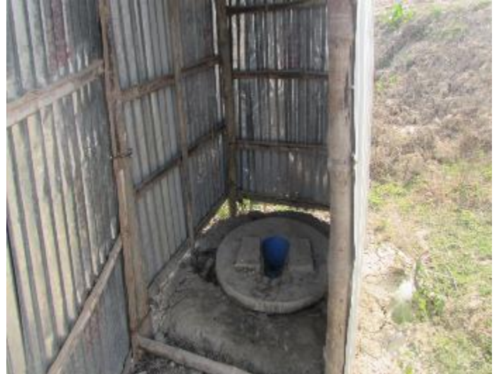
Latrine with no water seal
