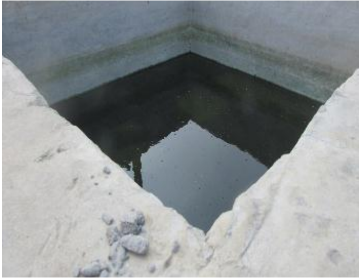
Water stagnant in the tank of worksite
