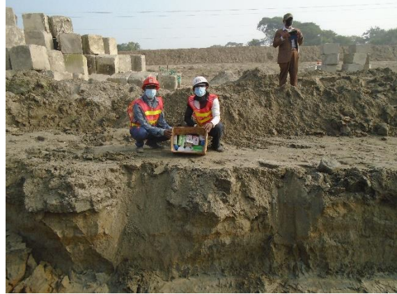
First Aid items for the workers at Slope protection work (Ch:31+450) under polder-48
