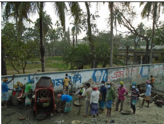
Workers without using PPE at Outlet-01 under polder-35/1
