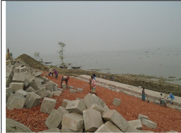
Workers without using PPE at Slope Protection Work (Ch: Km 4+239) under polder-35/1
