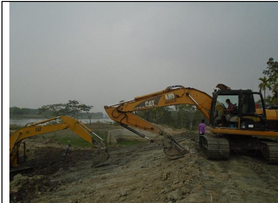
No signboard and demarcation at Embankment Construction (Ch: 50.05 km) worksite under polder-39/2C
