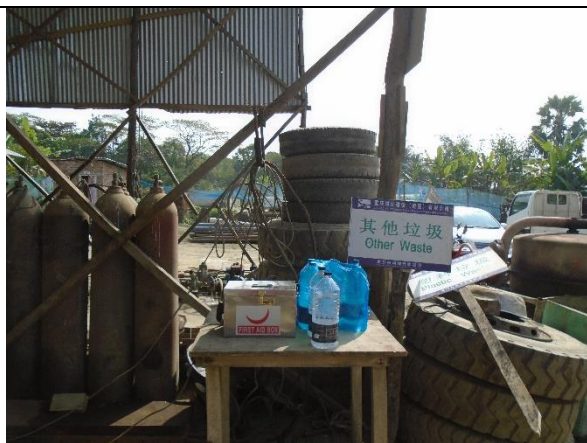
Supply of drinking water and First Aid box for the workers at Galachipa CC Block manufacturing yard under polder-43/2C
