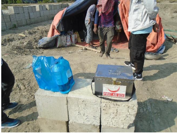
Supply of drinking water and First Aid box for the workers at DS-8 under polder-43/2C
