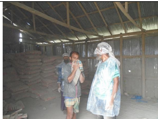
Workers work without PPE in Cement storeroom at Gulbunia CC block manufacturing yard under polder-41/1
