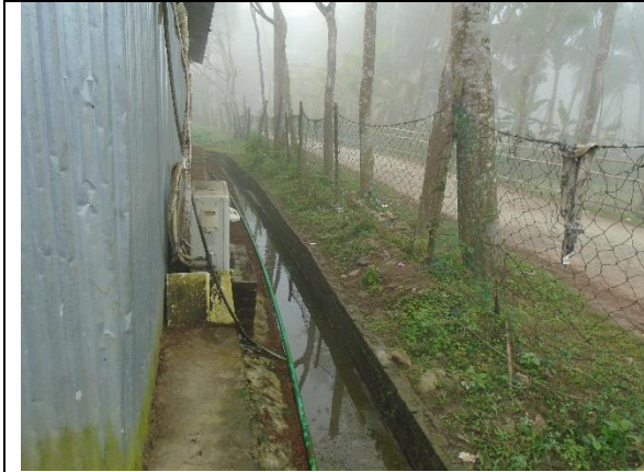
Stagnant water in drain at Burirchar CC block manufacturing yard under polder-41/1
