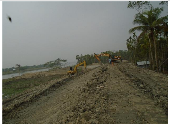
No signboard and demarcation at Embankment Construction (Ch: Km 50.05) worksite under polder-39/2C
