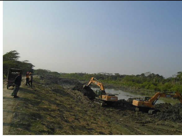
No signboard and demarcation at Embankment Construction (Ch: 0+850 km) worksite under polder-43/2C
