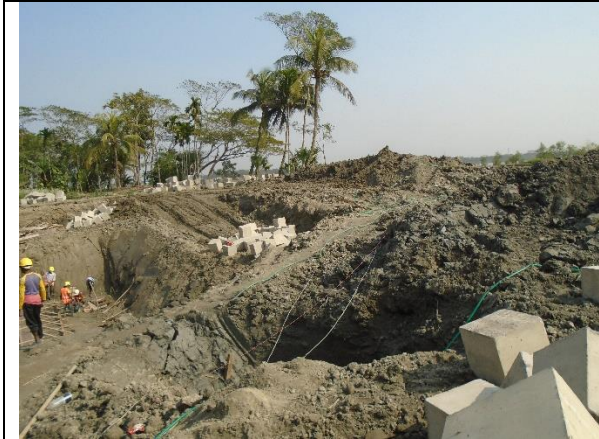
Electric wires haphazardly on the ground at the worksite (DS-8) under polder-43/2C
