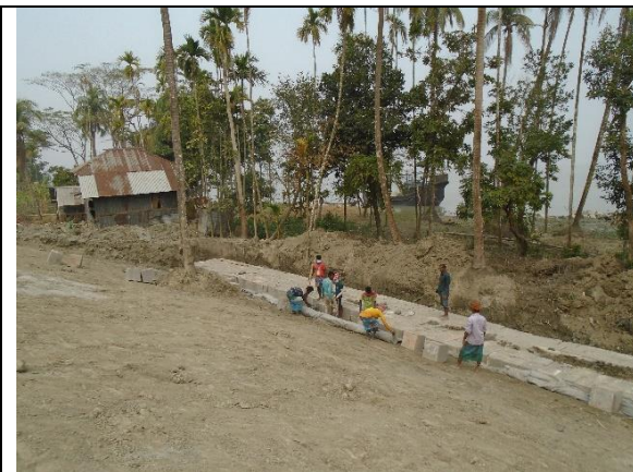
Workers without using PPE at Slope Protection Work (Ch: Km 3+880) under polder-35/1
