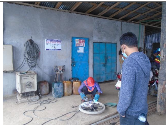
Workers welding work using proper PPE at Burirchar CC Block manufacturing yard under polder-41/1
