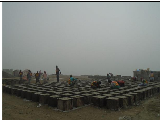
Workers work without PPE at Gulbunia CC block manufacturing yard under polder-41/1
