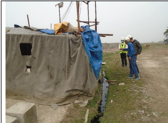
Stagnant water in drain at Nadmullah CC block manufacturing yard under polder-39/2C
