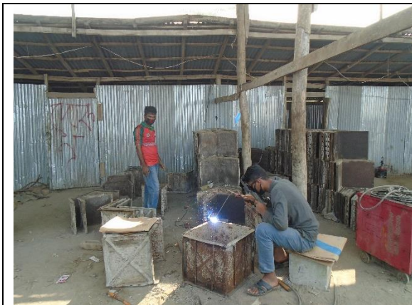
Workers welding work without using proper PPE at Dabluganj CC Block manufacturing yard under polder-47/2
