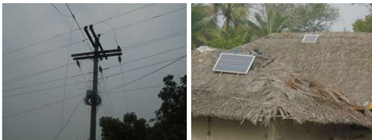
Photo 6.56: Electricity connections of the area
