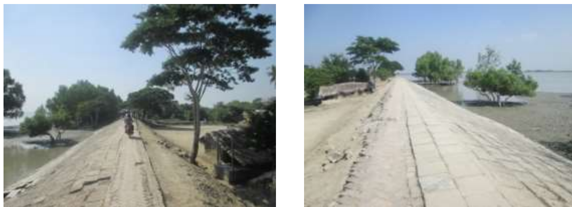
Photo 5-4: Present condition of existing slope protection work
