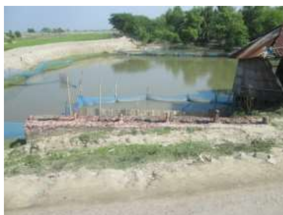
Photo 5-8: Deplorable condition of FS-9
