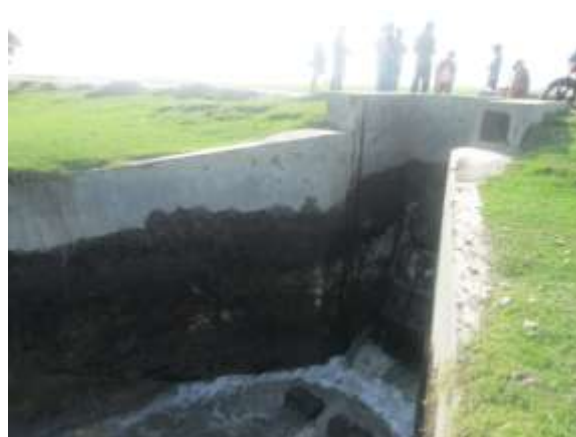
Photo 5-6: Moderately functioning condition of DS-2
