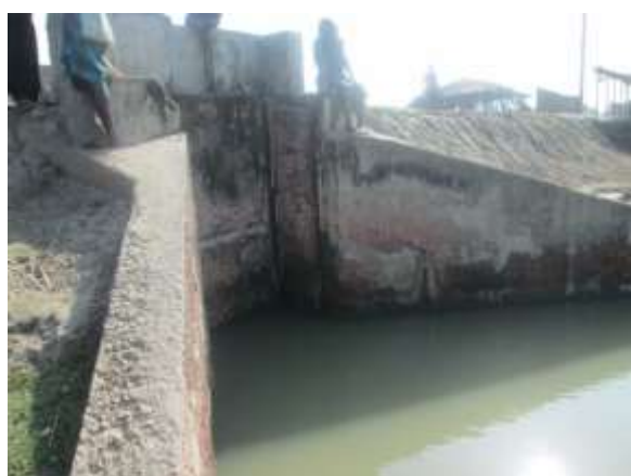
Photo 5-7: Moderately functioning condition of DS-3
