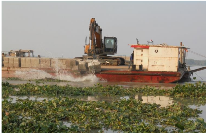
Figure 3-57: Dumping the CC block for the river bank protection works of Polder- 39/2C
