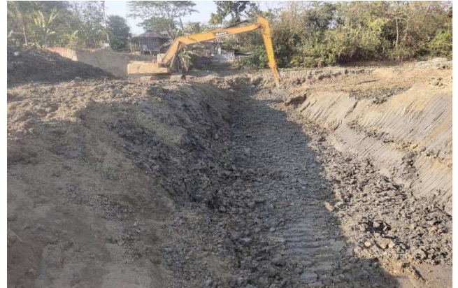
Figure 3-66: Excavating the foundation for DS-1 of Polder-41
