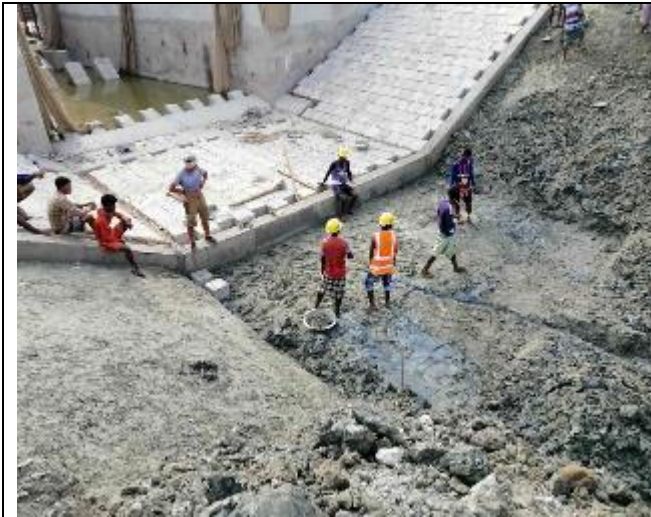
Figure 3-74: CC Blocks placing for loose apron (C/S) & slope of DS-01 in Polder 47/2
