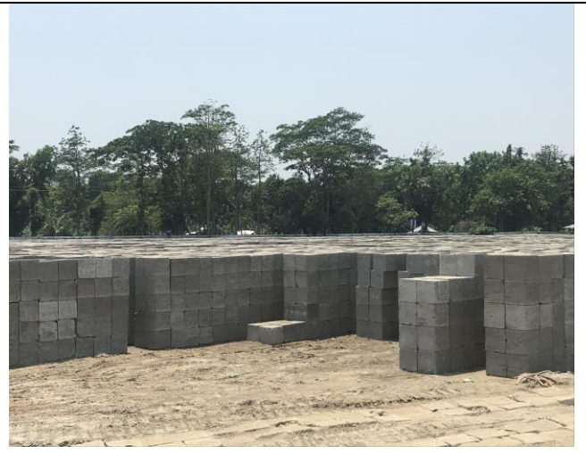
Figure 3-63: Manufactured CC Blocks piled at the permanent storing yard #A2 in Polder 39/2C
