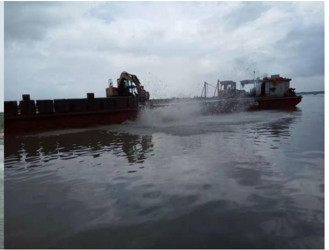
Figure 3-58: Dumping CC Block for river bank protection work (KM51+041-53+418) in Polder 39/2C
