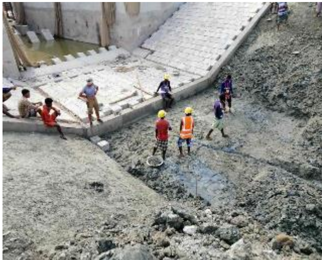
Figure 3-69: CC Blocks placing for loose apron (C/S) & slope of DS-01 in Polder 47/2
