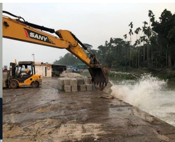
Figure 3-57: Dumping CC Block for river bank protection work (KM51+041-53+418) in Polder 39-2C
