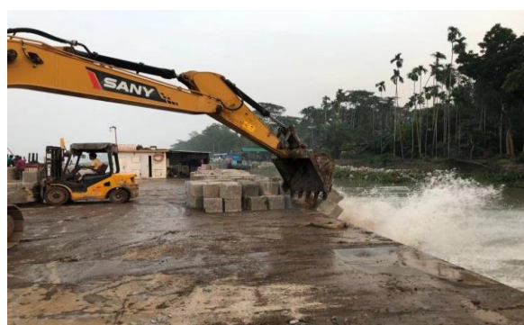
Figure 3-62: Dumping CC Block for river bank protection work (KM51+041-53+418) in Polder 39-2C
